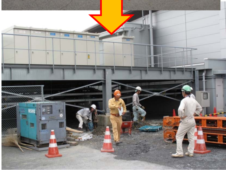
The bent stage was repaired. Power has been supplied to the RCS building.
